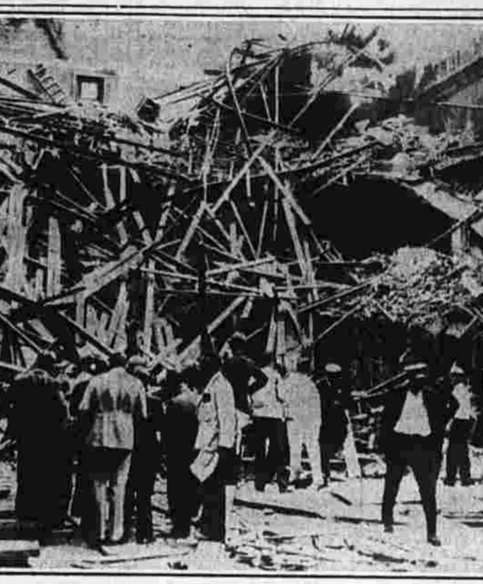
Death and injury claimed the last act of the famous Hollis Theater's history, two workmen being killed and twelve injured when the roof collapsed as the historic Boston structure was being raised.
